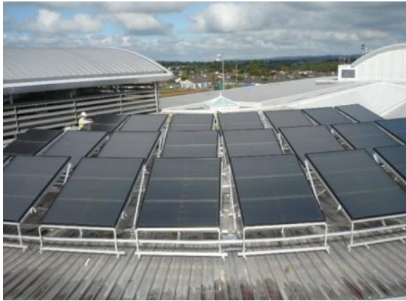
130 m 2 drainback solar water heater at Kilkenny Leisure Centre
